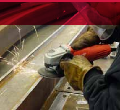
Smoothing the edges of roller coaster track with a resin fiber disc.
